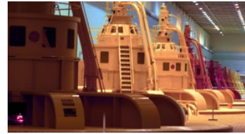
Hydroelectric Pump in Operation
