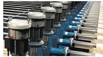
Vertical Pump in Operation
